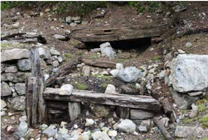
Verfallenes Mundloch. (Foto Rehm)
